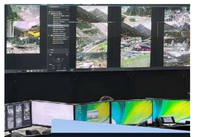
Srinagar Smart City Limited's Integrated Command & Control Centre is overseeing the Amarnath Yatra. The technology ensures safety, security, weather forecasting, traffic management, logistics, disaster management, sanitation and other service. (19 APR, 2021)
