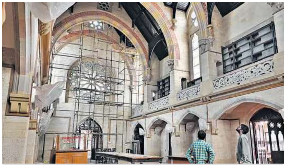
Revamp work in progress at the 160 year old Prayagraj Govt. public library
